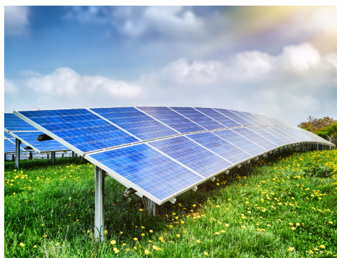
Solar Panel System
