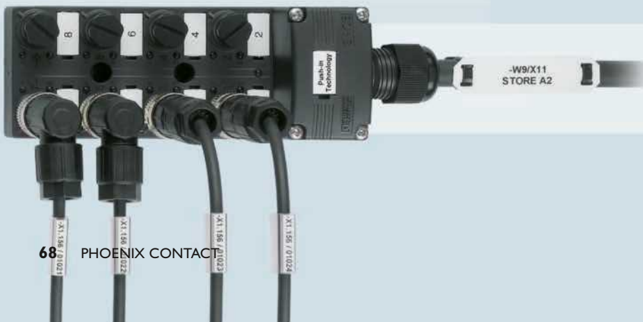
Field cabling with push-in connection
