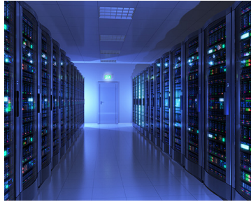
Data Center Solutions
