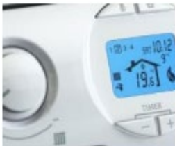
Boilers & Water Heating
