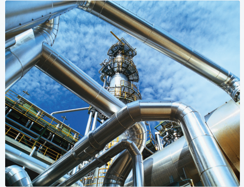
Chemical, Oil and Gas
