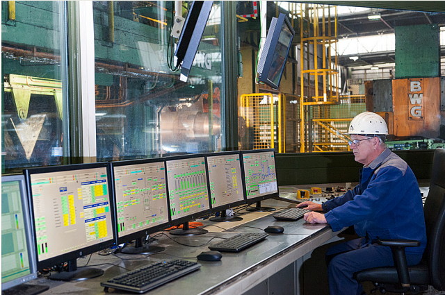
Reference: V7 control room
