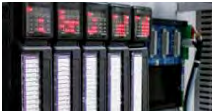
Connections to PLC
