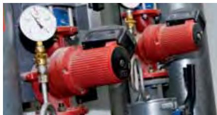
Actuators, valves, control cabinets
