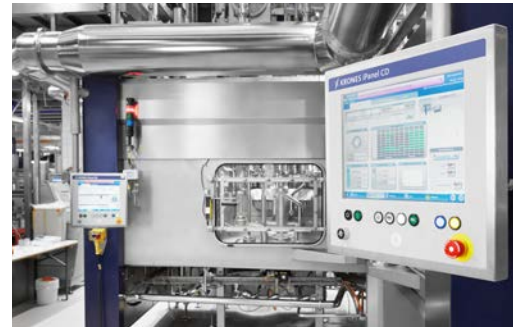
Control units with mixed technology solutions.
