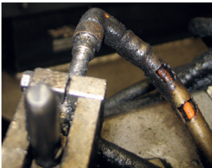
... but the durability was often compromised.
