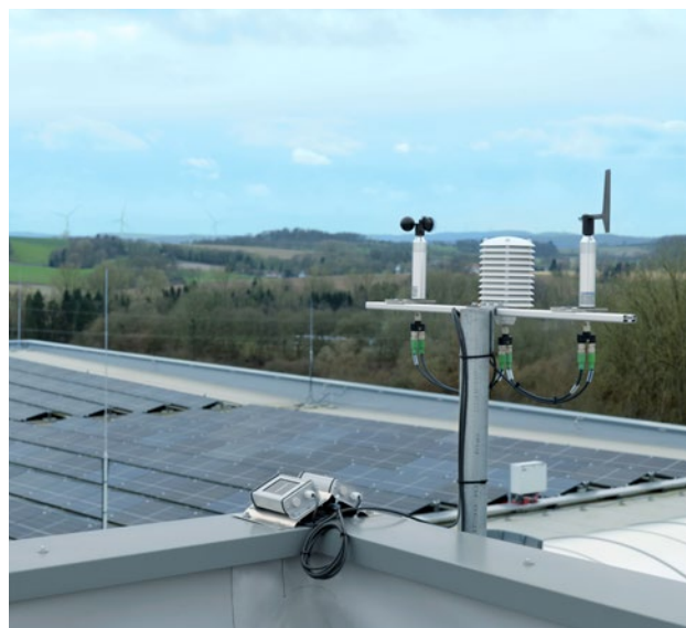
A sophisticated building control system works together with the energy management system
